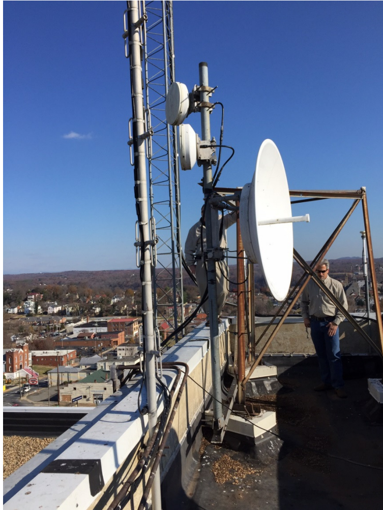
Figure 1: Three microwave dishes to be relocated to the new tower.
